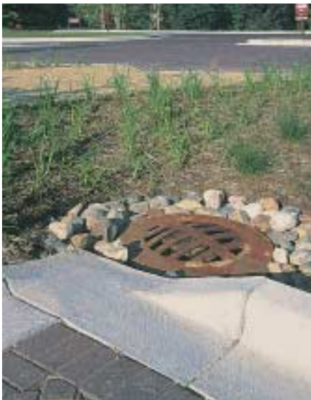
The design included drains to remove excess water generated from extreme rain events
