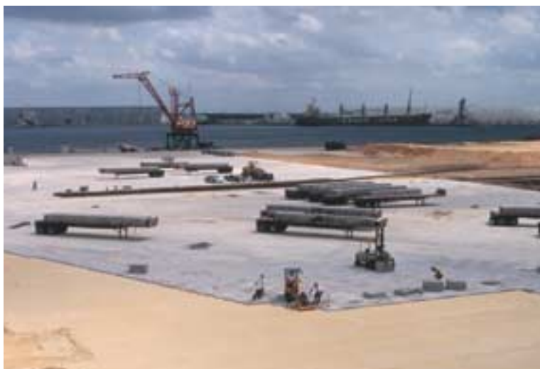
From 8,000 to 12,000 square feet of UNI-Anchorlock® pavers was installed per day using mechanized paver placement and sand screeding equipment
