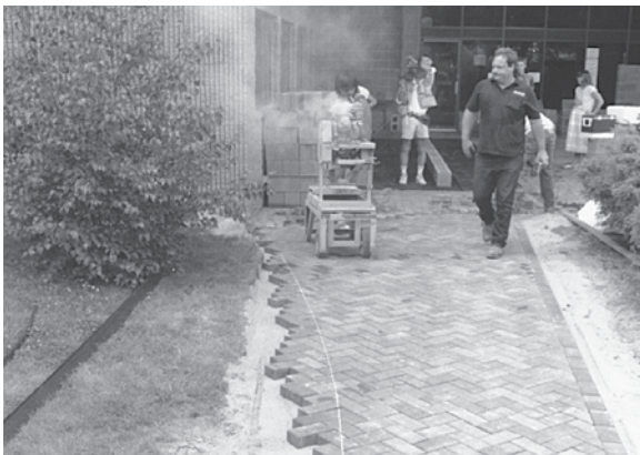
Figure 14. Saw cutting marked pavers on bedding sand. The cut pavers are carefully removed and edging is placed against the pavers and spiked in place.
